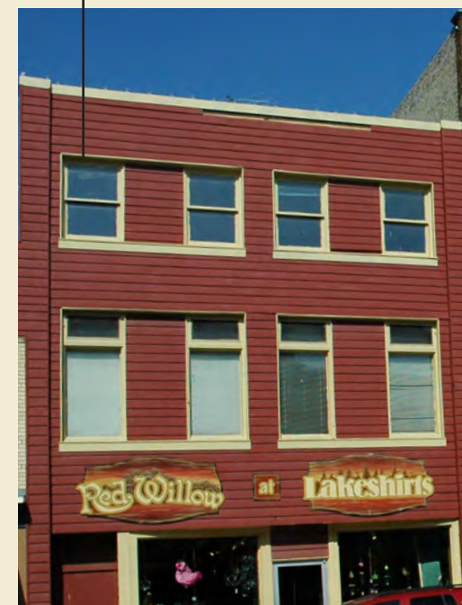
Inappropriate removal of cornice and facade
